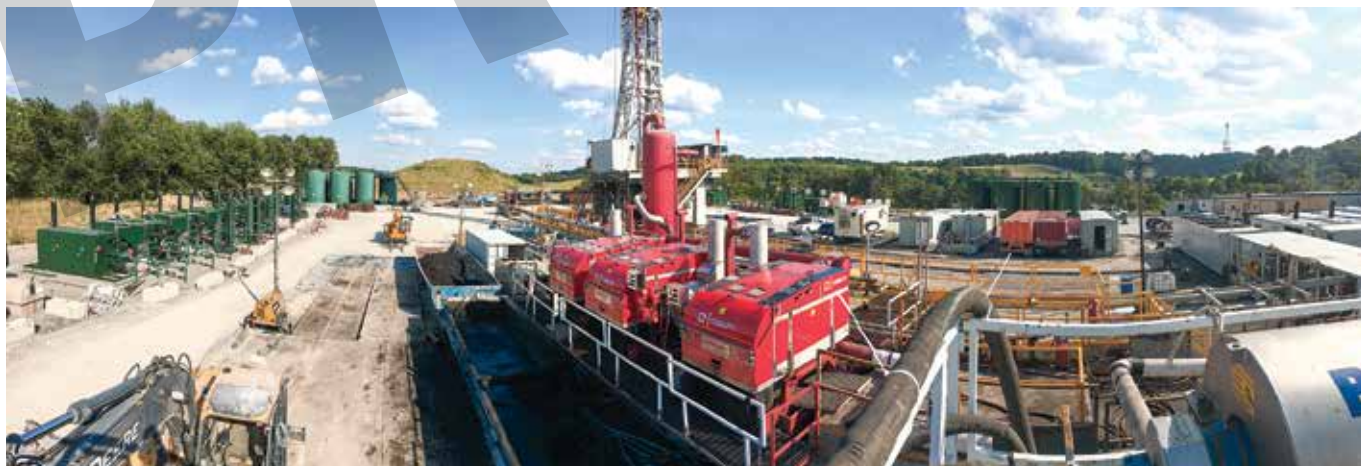
Fig. 1. In an industry first, the vacuum-based separation system was employed by EQT in the Marcellus shale.
