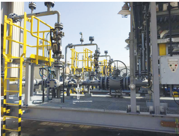
This image depicts a sampling connection of the Roxar modular meter at the inlet tree. (Source: Emerson Automation Solutions)
